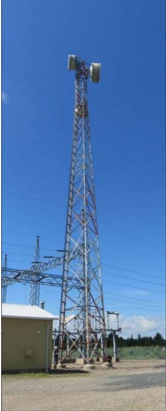
Photo 1: 30.48 metre, self-supporting steel tower with two microwaves and control building
